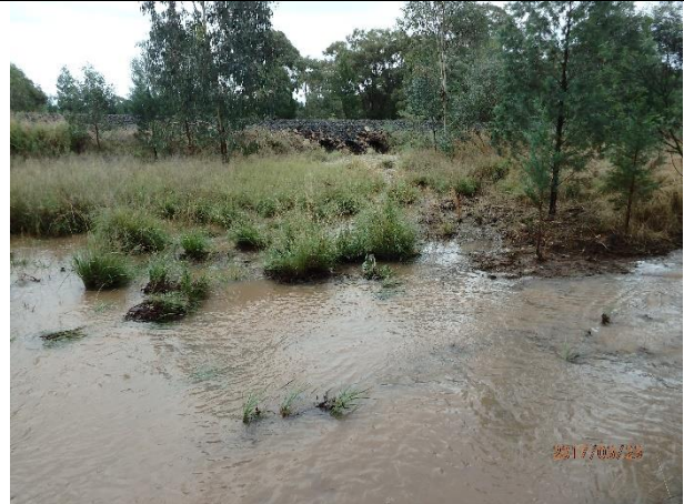
Plate C1.20 - Flooding on the unnamed lane that runs parallel to the railway to its south (Photo taken at 09:14 hours)
