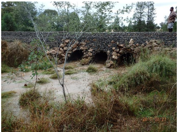
Plate C1.18 – Downstream side of the three 1050 mm diameter corrugated pipes beneath the railway to the east of Haynes Street (Photo taken at 09:12 hours)
